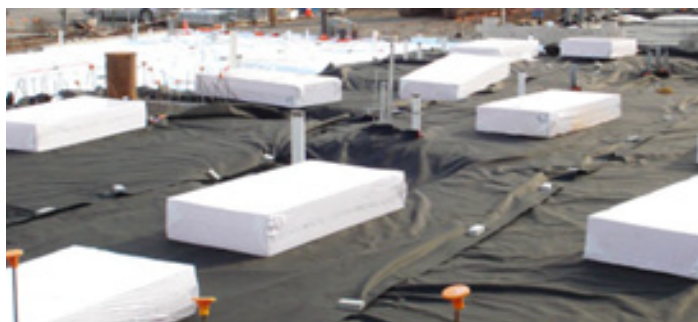
Figure 8. Standard vapor barrier with unsealed seams.
