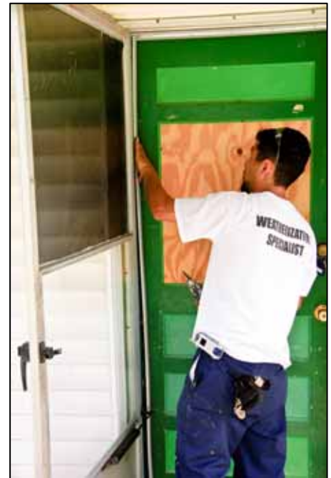
A weatherization specialist with Houston's Sheltering Arms, funded through TDHCA's Weatherization Assistance Program, applies weather stripping to a low-income Texans' home.
